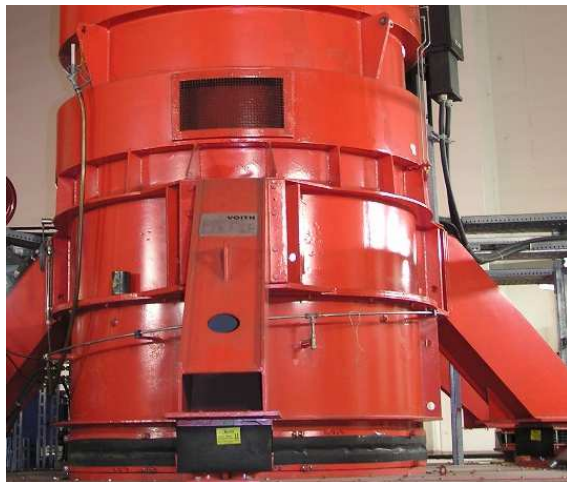
Exhaust air ventilator A1 in the exhaust air station
