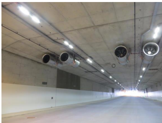
Jet fans above the lanes
