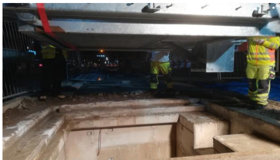
Shaft cover flap assembly ready to be installed in the recessed area in the tunnel ceiling at the platform
