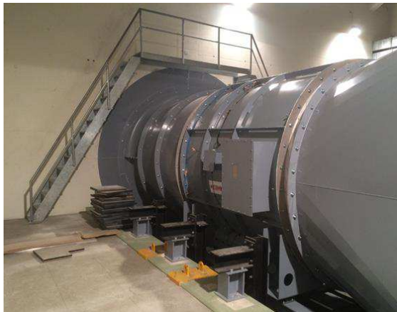
Axial fan for longitudinal ventilation (Saccardo nozzle)
