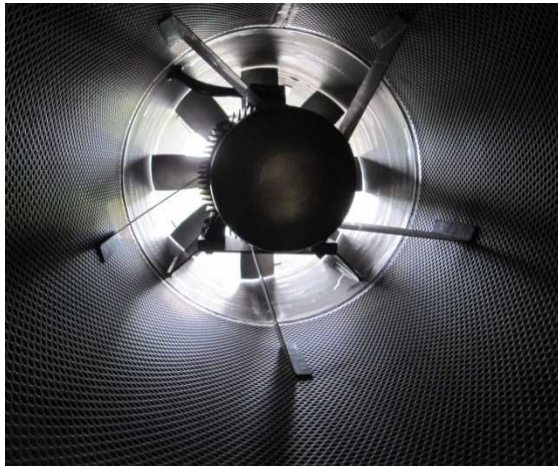
Technical installations in the tunnel
