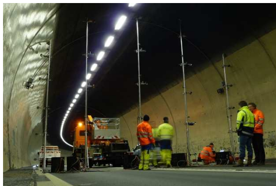
Measurement grid installed for tests and calibration of air velocity monitors
