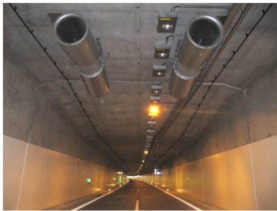
Jet fans with attenuators slanted by 7°
