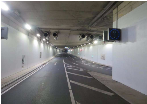
Access with jet fan group in the Kö-Bogen Tunnel
