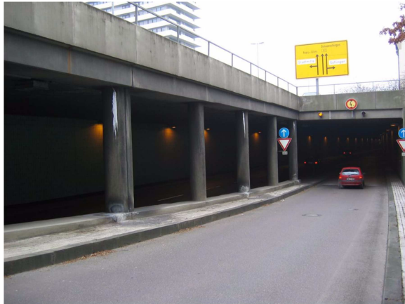
Covered Road Section and Entry Portal of the Bismarckring Tunnel in Ulm
