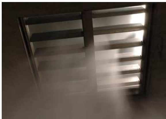
Exhaust dampers in the false ceiling: air extraction in normal operation or smoke extraction in case of tunnel fire
