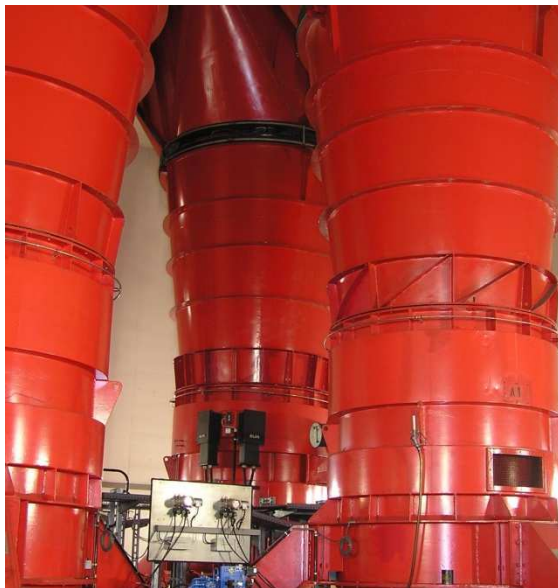
Axial fans in exhaust ventilation station
