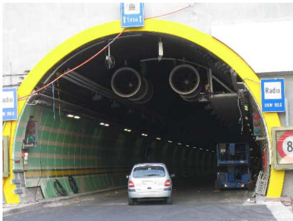
Jet fans at northern portal of tunnel Berne/Lucerne
