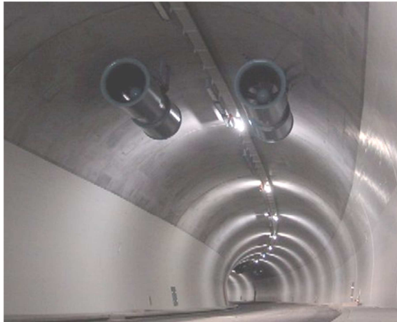
Jet fans at southern tunnel portal
