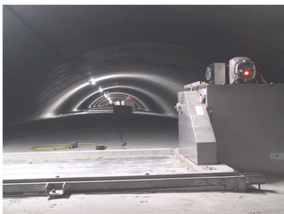
Ventilation duct with remotely controlled dampers
