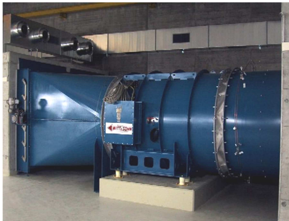
Exhaust fans for normal and emergency operation
