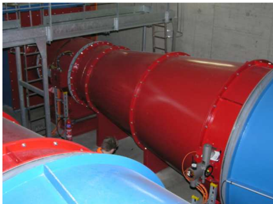
New exhaust fans for smoke extraction "Kniebrücke"
