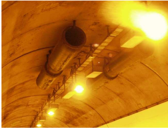
Jet fans before the refurbishment
