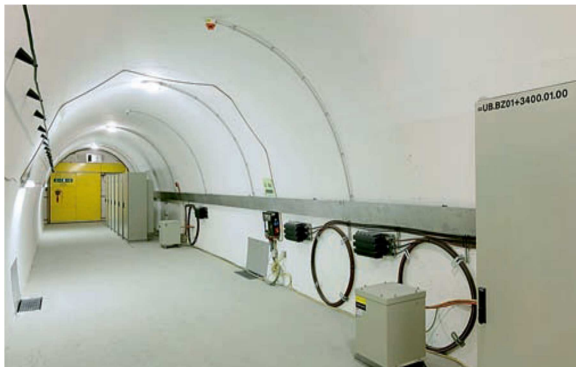
Standard electrical cabinets for housing of different electrical equipment in a cross-passage
