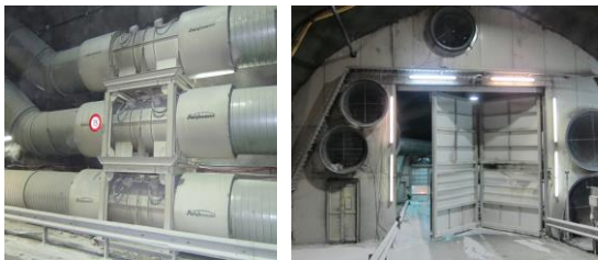
Site ventilation system and lock system in the access tunnel and ventilation shaft
