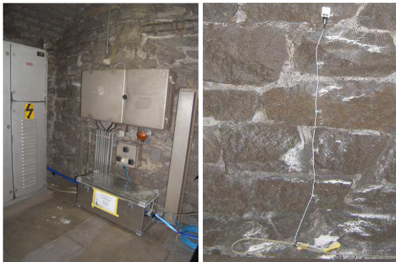
Installation inside of the cross-passage for data acquisition (left)
