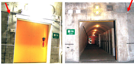
Pressure transducers (red marks) to record the train-induced pressure variations in the rail tunnel
