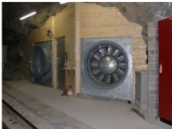
Air extraction with axial fans from the Jungfrau railway tunnel
