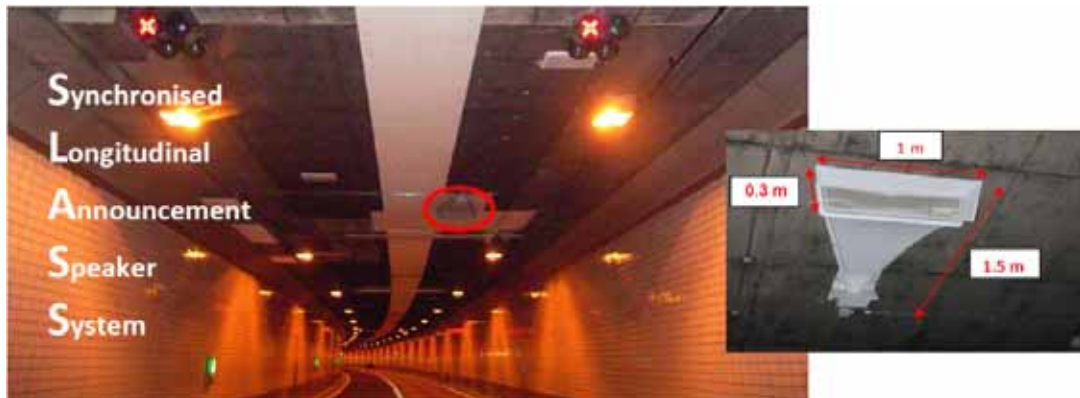
Figure 1: Illustration from [13] of SLASS loudspeaker system in the Elbe tunnel.
