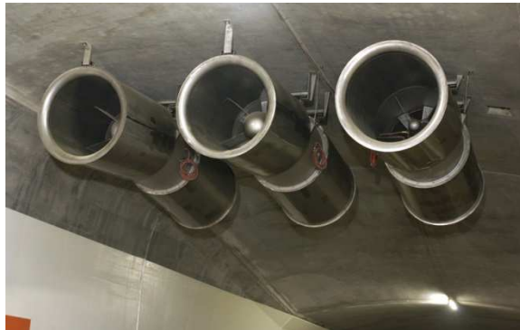
Jet fan installation in a ceiling niche Kirchenwald
