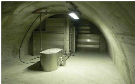
Isolation damper in ventilation ducts between west- and eastbound tunnels Kirchenwald
