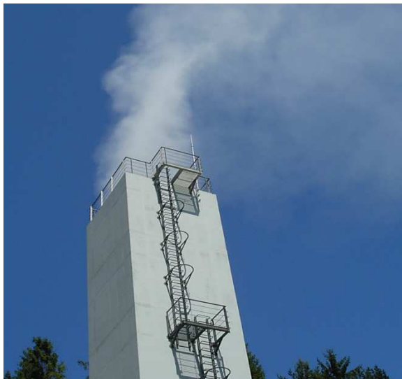
Exhaust shaft during smoke test in tunnel
