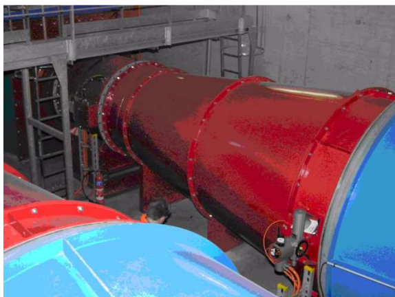
New exhaust fans for smoke extraction "Kniebrücke"
