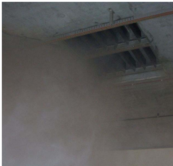
Fig. 15 Non-toxic smoke extracted through the extraction damper in the Flüelen túnel (Switzerland)
