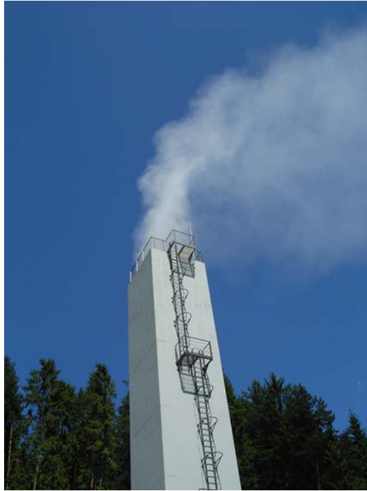
Fig. 14 Smoke exiting the exhaust shaft
